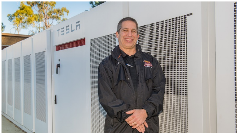
Figure 3- Campus Energy Manager Kenny Seeton in front of 20 Tesla batteries providing 1MW/4hr of peak energy reserve storage for the campus.
