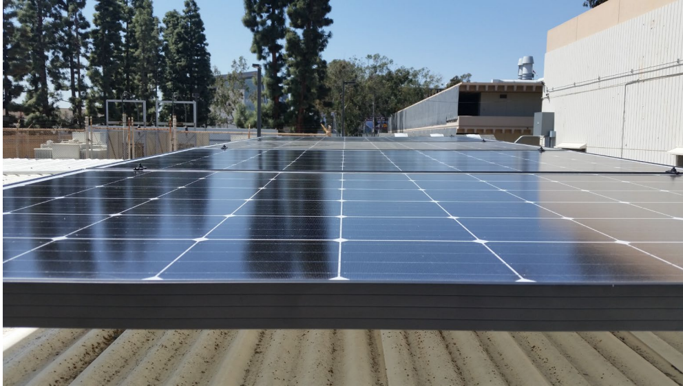
Figure 8- Solar panels powering the campus Net Zero Innovation Center.
